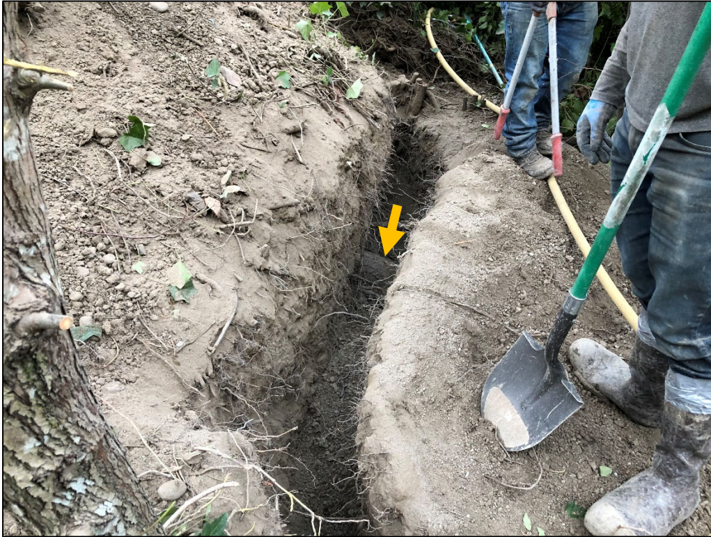
Photograph 1. Arrow indicates the location of the ten inch root within the excavation zone. The base of tree 7 is just outside of the frame in the top left corner.
